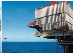
HVDC Light Module on Troll-A platform (ABB)
