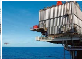
HVDC Light Module on Troll-A platform (ABB)
