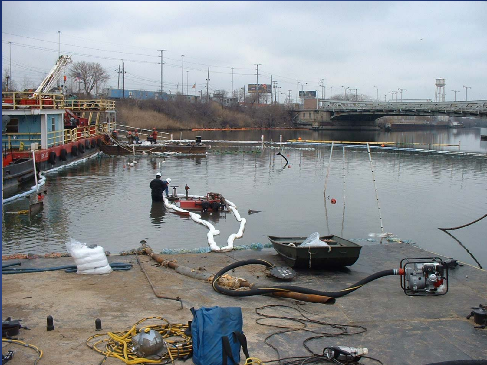
Photo taken from the exposed bow of the barge, with the stern ~295' to the rear and under ~20 feet of water. At this point, all oil is thought to remain on board.
